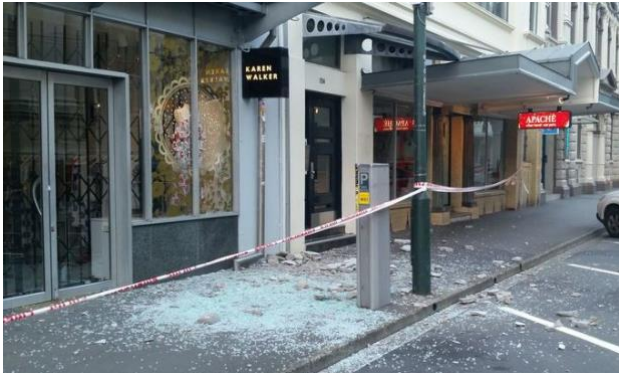
Figure 2: Illustrating exterior damage to non-structural elements observed in the Kaikoura earthquake (from Radio NZ/Susie Ferguson)
