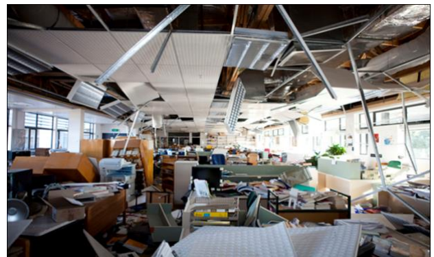
Figure 1: Illustrating damage to non-structural elements observed in the Canterbury earthquakes (from Dhakal, 2010)
