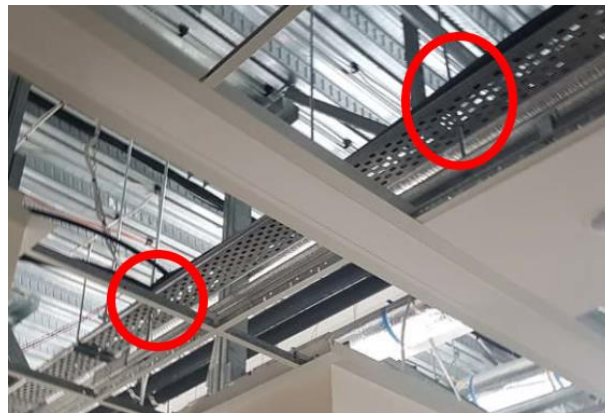
Figure 4: Ceiling hangers run through cable tray
