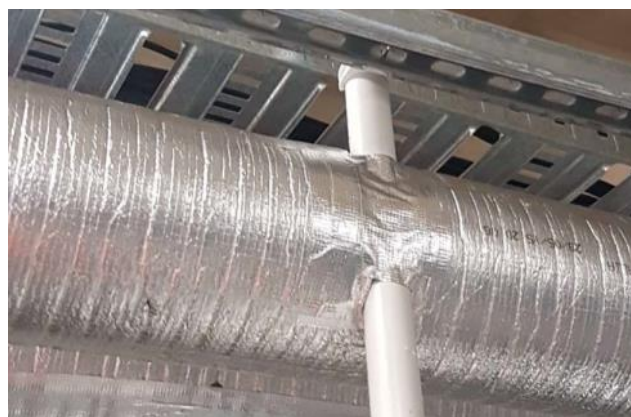
Figure 5: Clash of pipe with insulated pipe and cable tray
